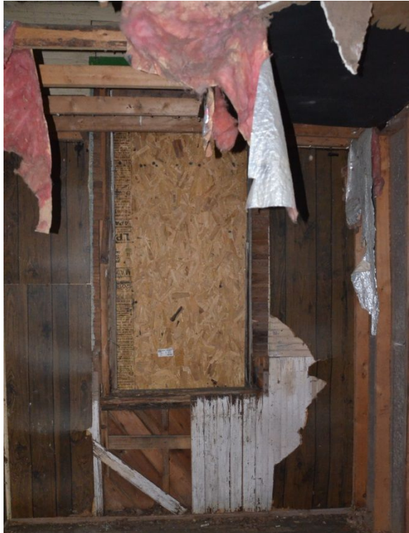
Image 6. Empty southernmost window frame in western wall of the 1927 classroom. Photo by Grace Abernethy.
