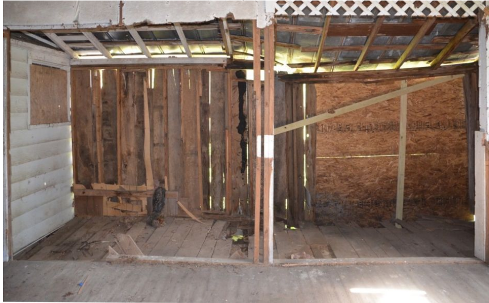
Image 18. North wall (missing) of 1940s classroom. Photo by Grace Abernethy.
