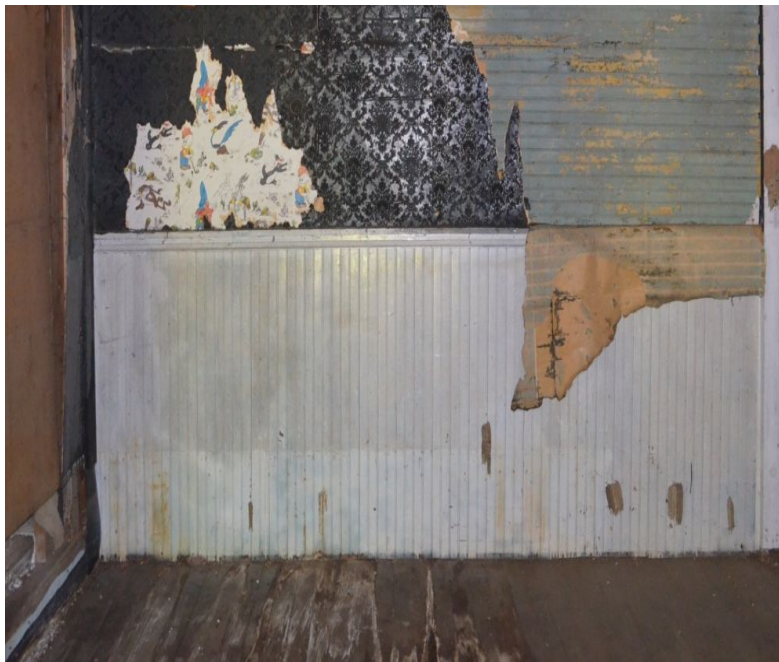
Image 8. Deteriorated floorboards in the southeastern corner of the 1927 classroom. Photo by Grace Aberenthy.
