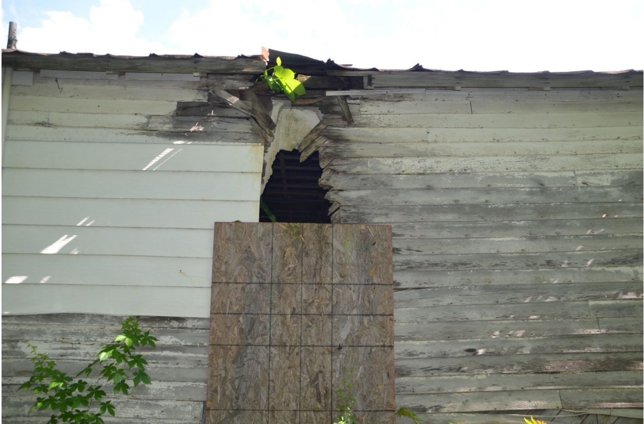
Image 16. Fissure in south wall of 1940s addition. Photo by Grace Abernethy.
