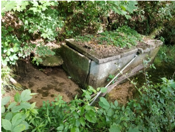
Figure 6-29. The secondary spring, once called Cleveland Spring. The casing once containing the spring water has failed. Courtesy of the author.
