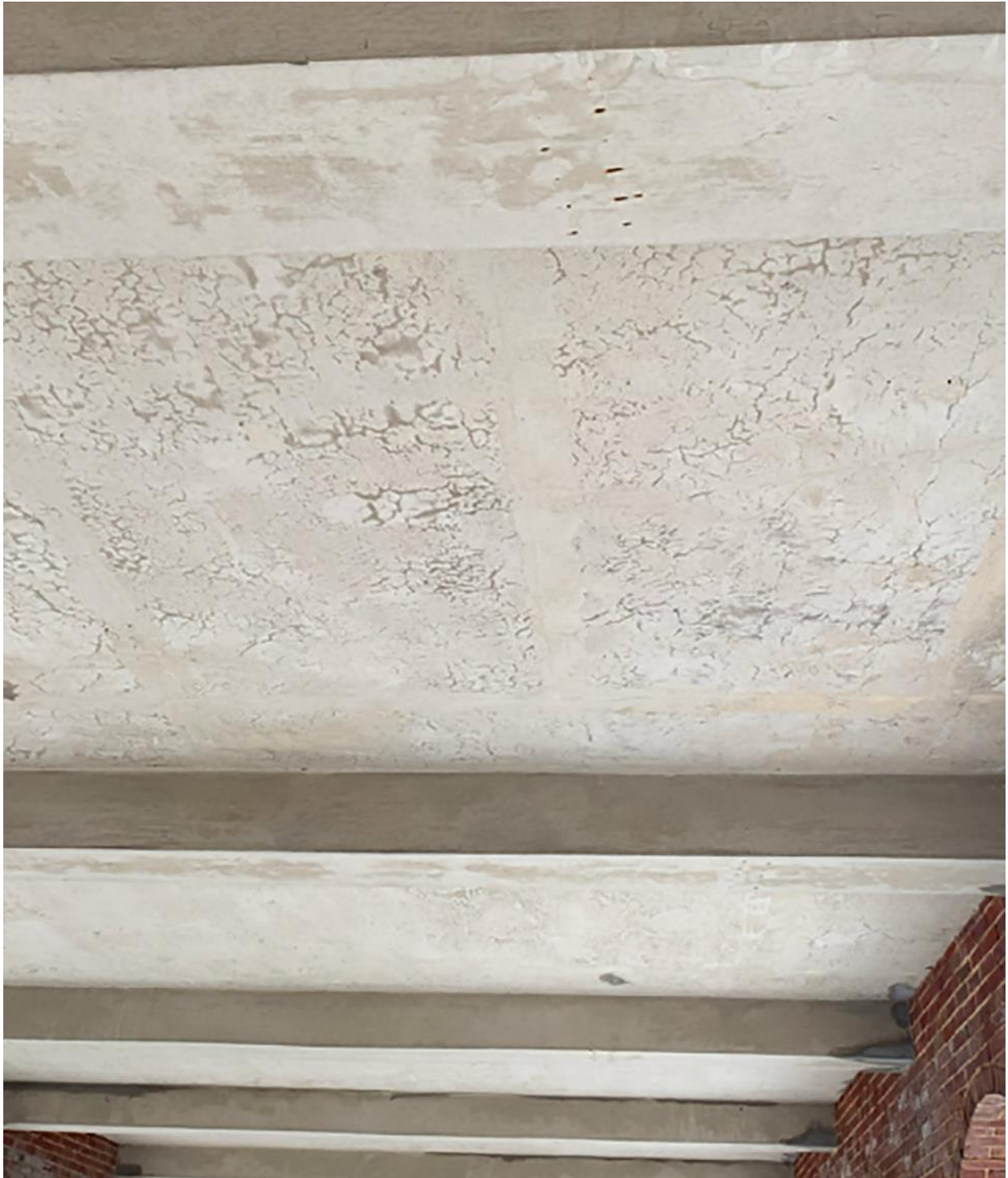
Figure 40. Damage of sleeping porch ceiling
