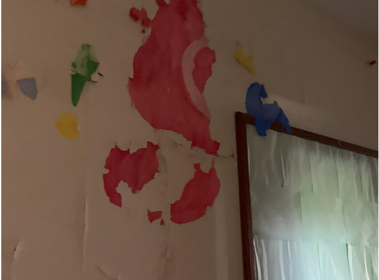
Figure 28. Cresson White paint peeling revealing children's mural underneath
