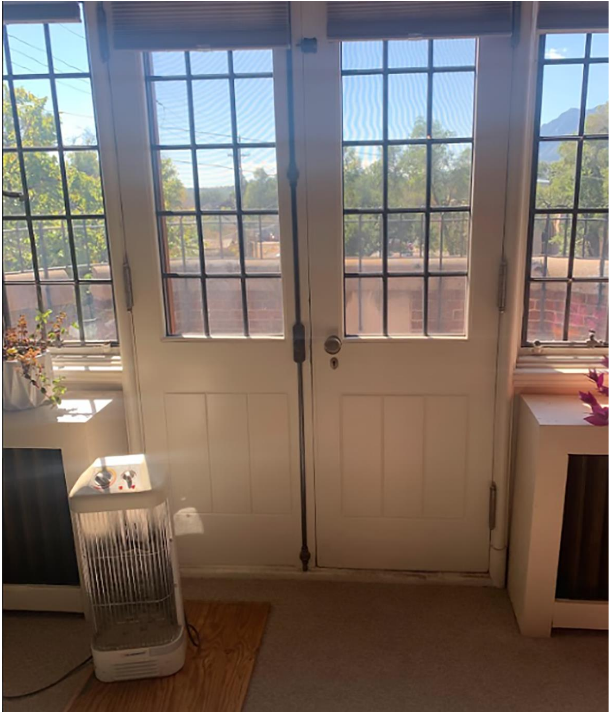
Figure 59. Doors leading to sleeping porch - blocked off
