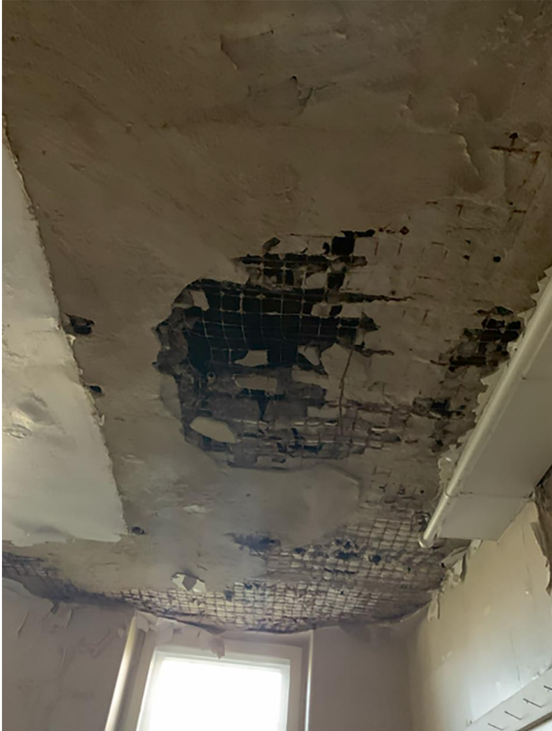
Figure 27. Ceiling damage of Maple House
