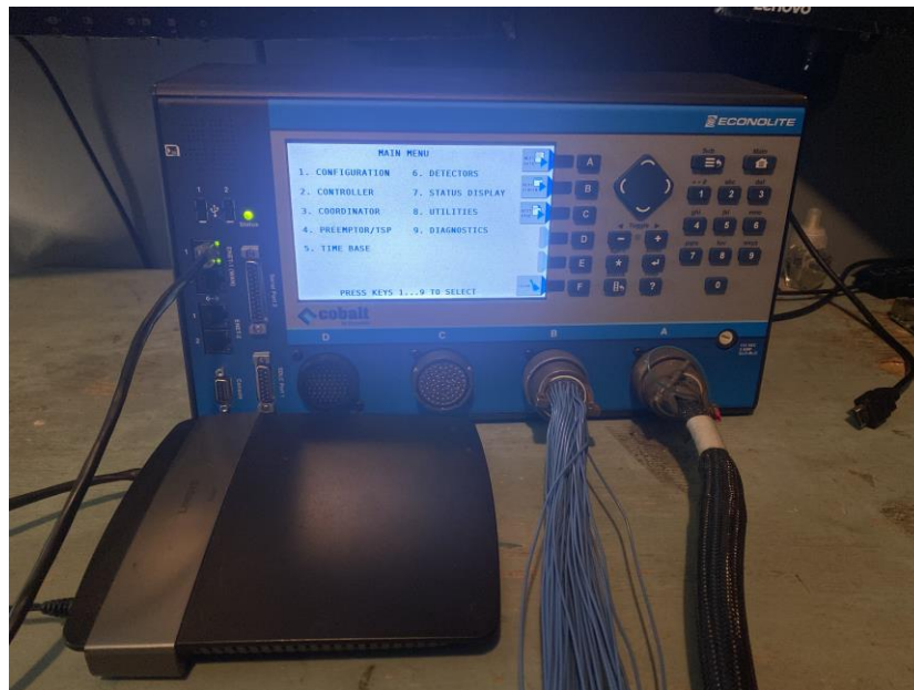
FIGURE 5-1 A CLOSE-UP OF THE ECONOLITE COBALT TRAFFIC SIGNAL CONTROLLER.
