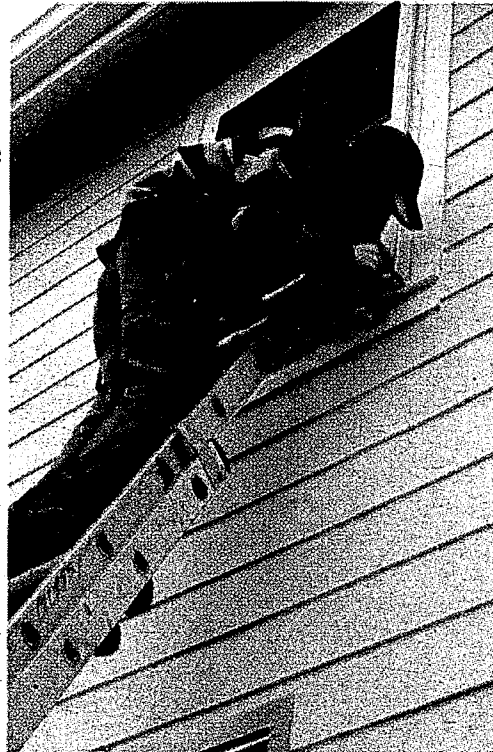
Chuck Redden of Glazier Windows helps complete restoration work on the new Chi Omega house. The house was originally the Pi Kappa Alpha fraternity. Photo by Emily West
