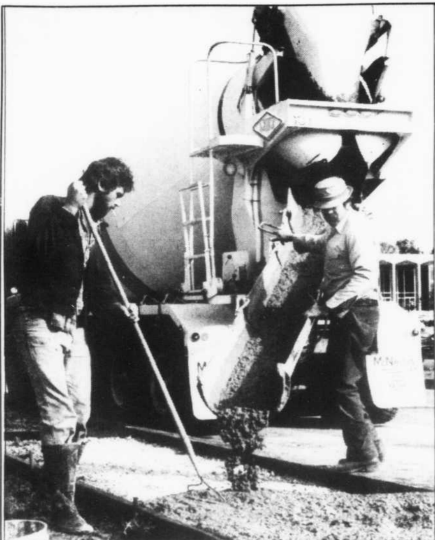
Capital City Contractors employees Johnny Gidcomb (left), who is mayor of Hasbarg, and Butch Dabbs pour concrete for the sidewalks along the west side of the loop.
